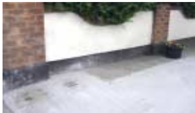
Damage to garden wall
