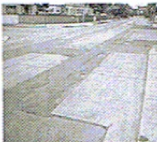
No funds to resurface this section
